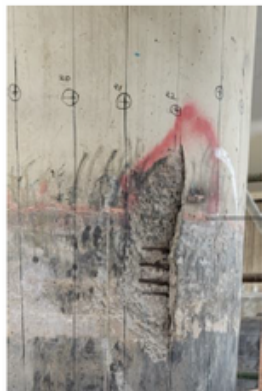
Photo of Column 5 with spalled concrete
